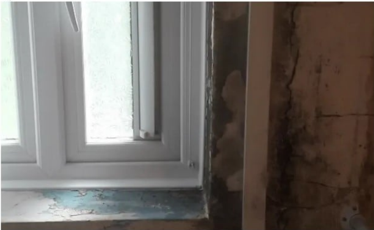
This social housing for local residents was full of damp and mold GB news
